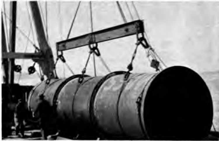
84" U. S. Cast Iron Pipe Outfall Sewer being installed by Metropolitan Sewer and Water Board, Boston, Mass.
